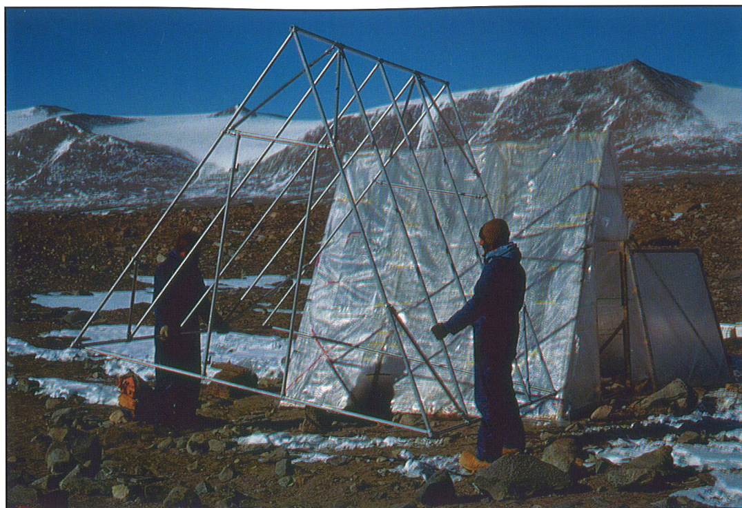
Erection of greenhouses in the vicinity of the Canada Glacier SSSI (before its establishment) for experiments with flowering plants from New Zealand. The importation of non-indigenous plants and animals into Antarctica is now restricted by permit under the terms of the Madrid Protocol and there is an increased awareness of the need to protect the Dry Valleys as much as possible from introduced species, including microbiota.
